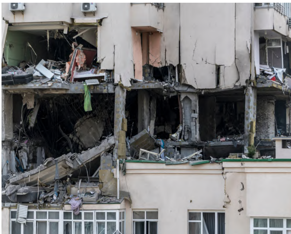
Much of the apartment building's 18th floor was destroyed.
